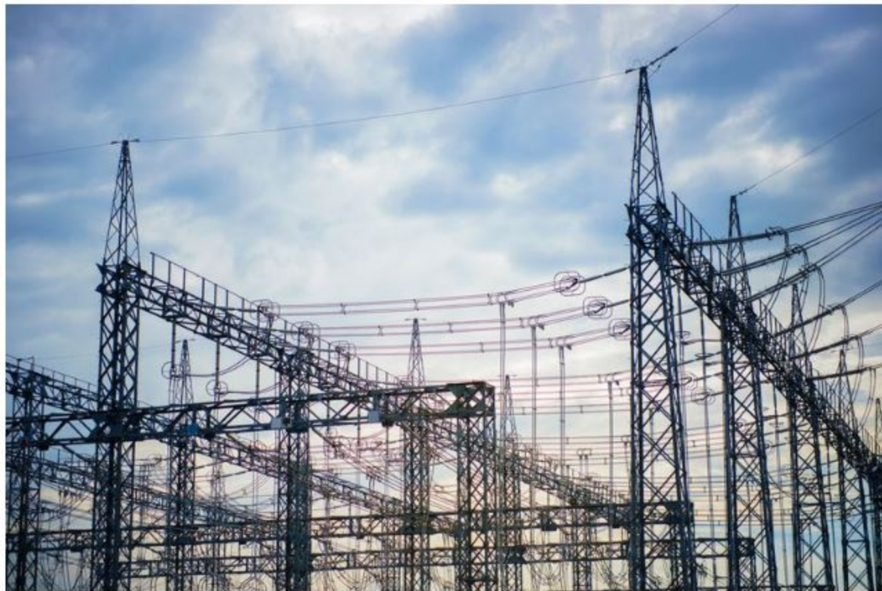
Getty image of an energy facility. (Image: Lincolnshire Live)
